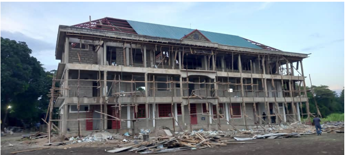
Progressive transfer of Usa Seminary to the new site: offices, classrooms and examination hall on the second floor
